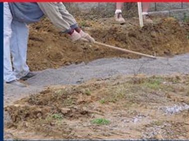
(2) Rock foundation & leveling pad. Crushed rock is placed 2 to 4 inches deep in trench and leveled.
