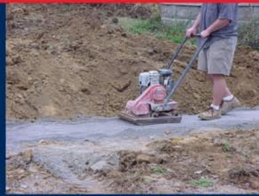
(3) Foundation and leveling pad is completed with a mechanical plate tamp or hand tamp.
