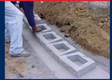
(4) Base course of Geostone blocks are placed on compacted level rock foundation.
